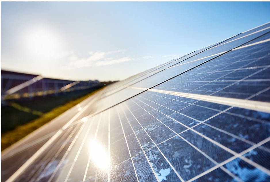
Symbolfoto „hep-Solarpark“ (credit: hep)
